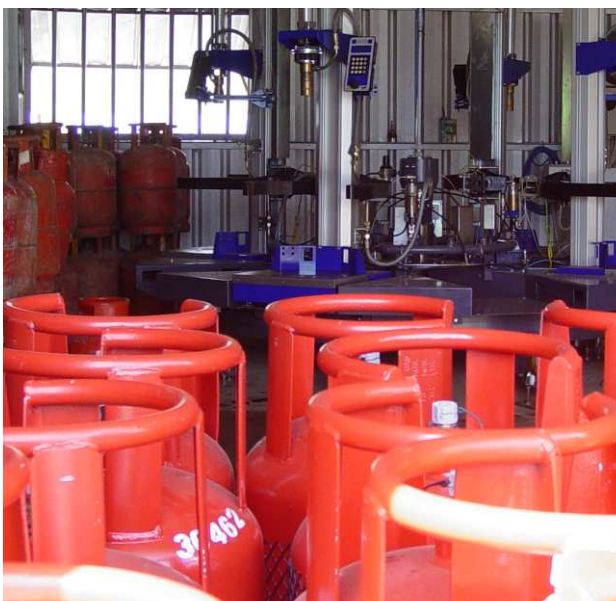
Maldivian Gas Plant
