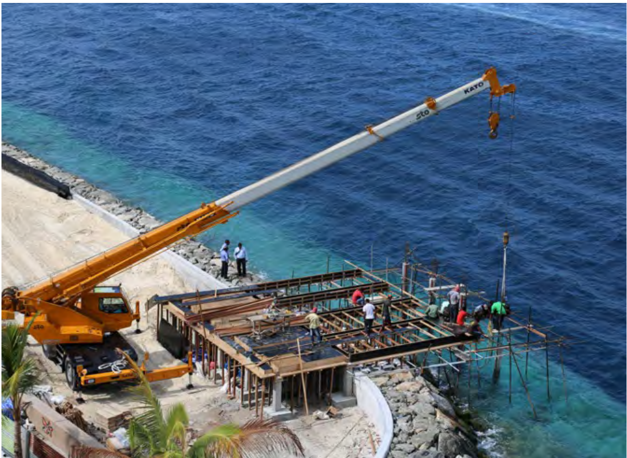
Photo: Construction of Fishing Pier at Male' West Coast – a project by State Trading Organization Plc
